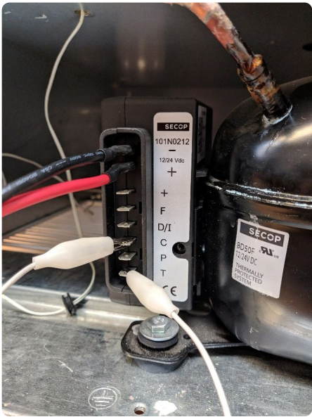
A jumper wire joining the C and T terminals on a Secop controller.
